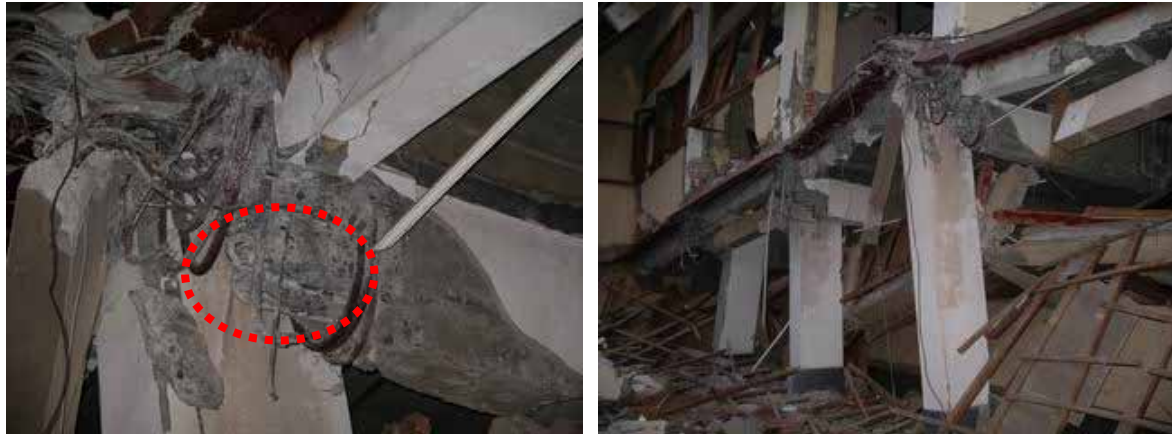
University of Economic Science (STIE) / Beam bottom rebars inadequately anchored to joints
