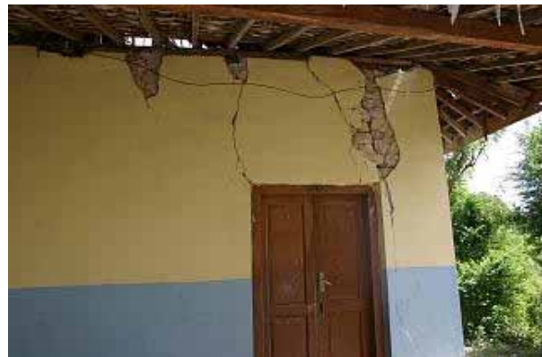
Damage to corner wall
