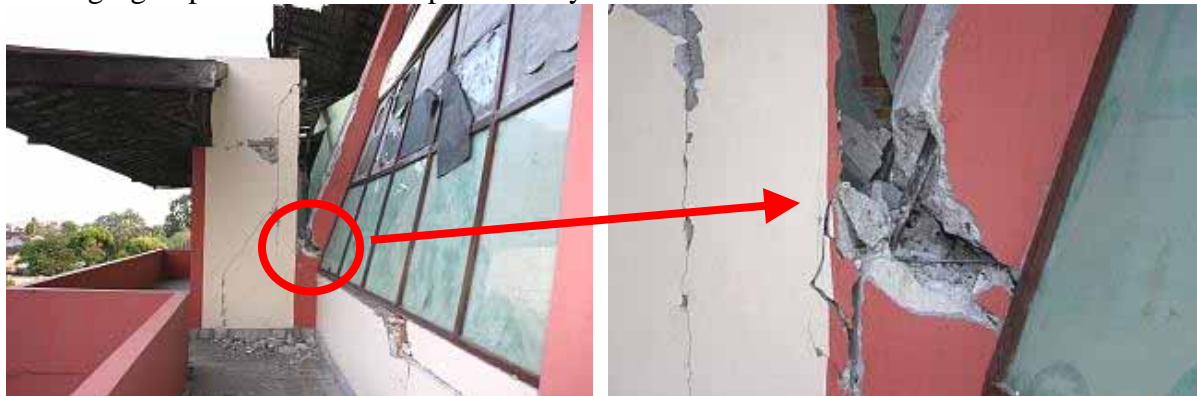
Heavy damage to RC columns and exposed rebar
