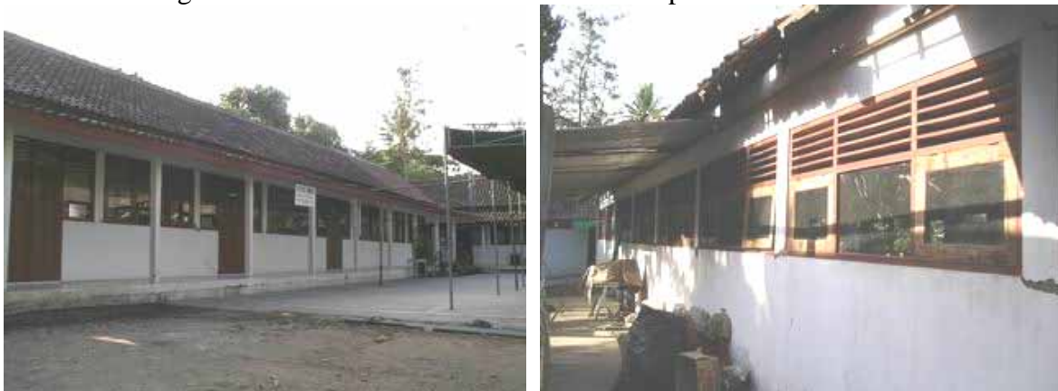
SLB-PGRI Trimulyo / Cracks found in column ends
