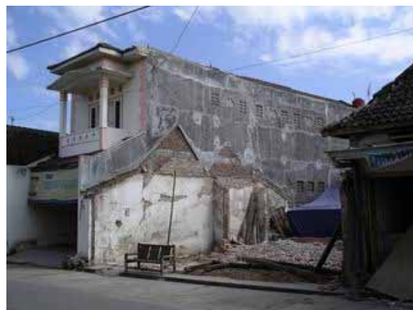
Survived house with URM and RC frame
