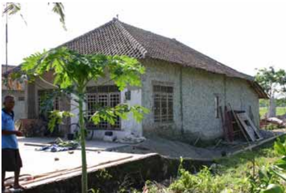
Stone masonry house with cracks in walls
