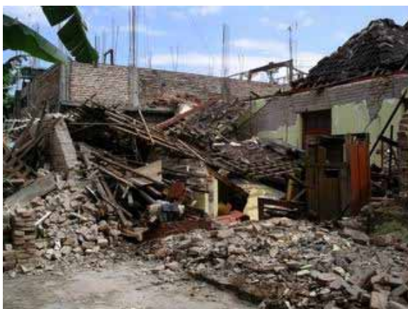
Devastated URM house
