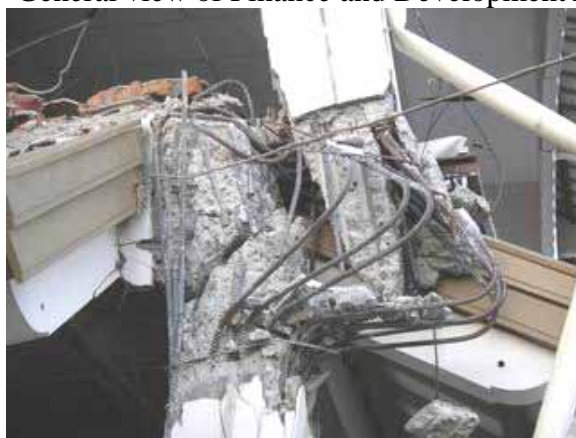
Beam-column joint failure
