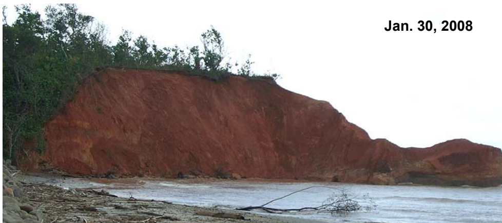
Fig. 2. Exposed slip surface of laterite (Location 3^{\circ}25'38.5''\text{S} , 101^{\circ}53'51.4''\text{E} ): The photo above was taken on Oct. 6, 2007 by O. Aydan, while the photo below shows the same surface four months later (photo by K. Konagai). With its toe being washed by sea waves, the slope has been eroded slightly inland. See some trees on slopes have disappeared.
