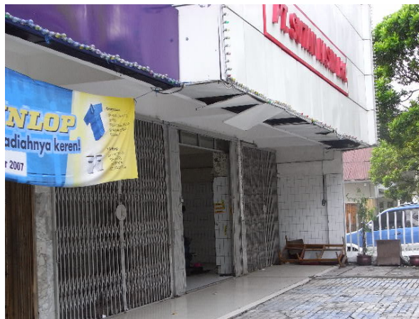
Fig. 10. Ceiling boards are still left damaged 4 months after the last event.
