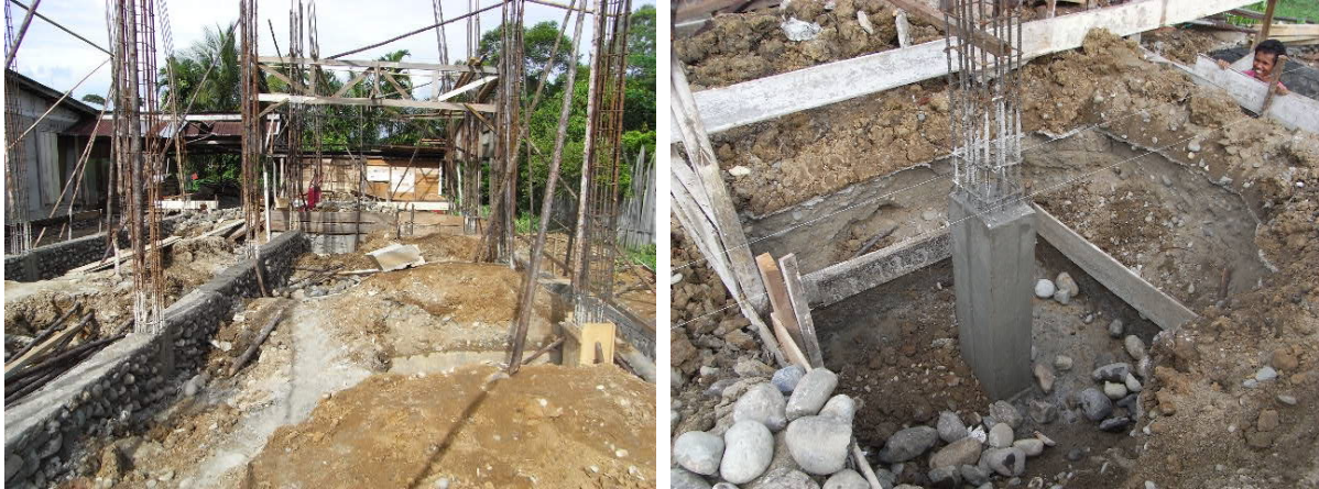
Fig. 7. Unreinforced foundation beams are provided only in the longitudinal direction (left). Column reinforcement needs to be properly embedded into footing slab to form a rigid foundation system (right).
