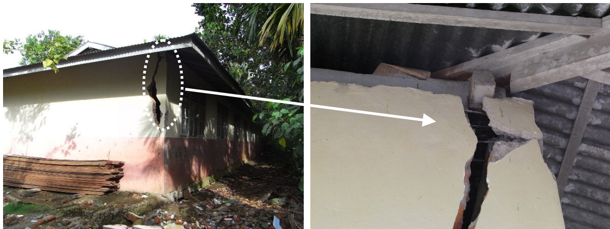
Fig. 5. Damage to URM wall due to pull-out failure at collar beam joint.
