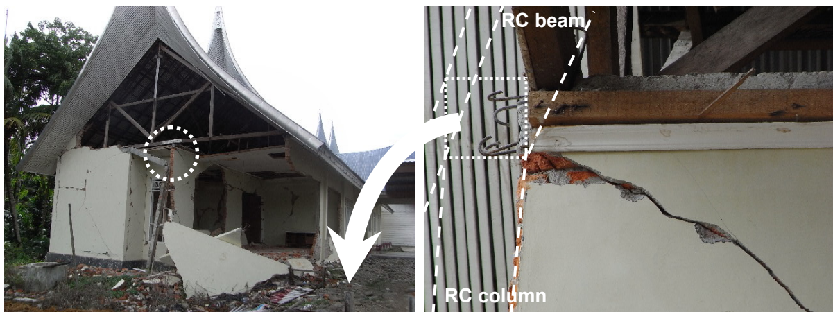
Fig. 6. Out-of-plane failure of URM wall due to pull-out failure at beam-column joint.
