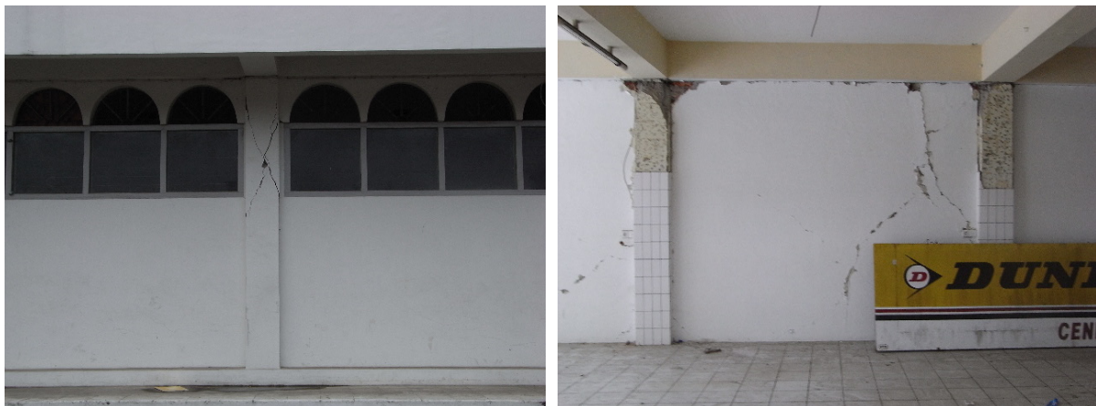
Fig. 8. URM walls are contributing to column shortening and lateral force resisting mechanism.
