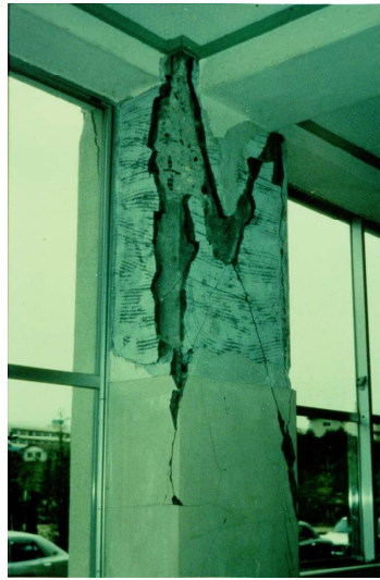
Damage class III: (left) Crack width about 2mm on structural concrete (right) Spalling of covering concrete and rebar slightly exposed
