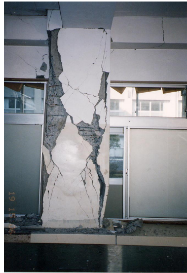
Damage class IV: Rebars exposed but their buckling/fracture not observed
