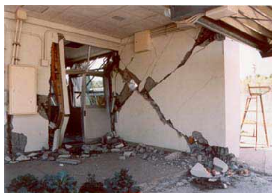
Damage class V
