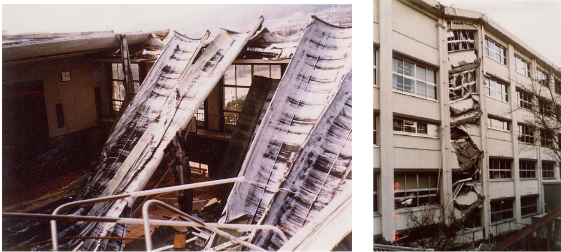
Photo 1: Seriously damaged schools (1995 Hyogoken-nambu earthquake, AIJ 1997)
